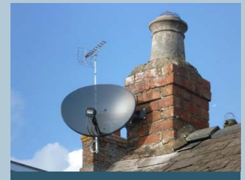
Figures 60 & 61: There are various threats to the conservation area including modern kerbing materials and satellite dishes.
